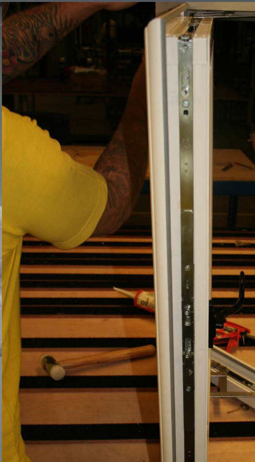
high security ironmongery used throughout
